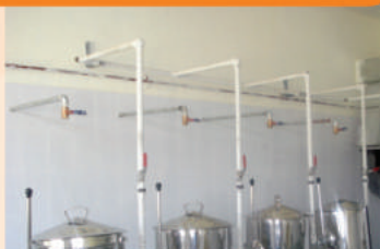
STEAM PIPE LINE
